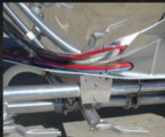
Wiring and Airline Accessibility
