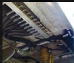
Central Grease Block and Floor Drain Valve
